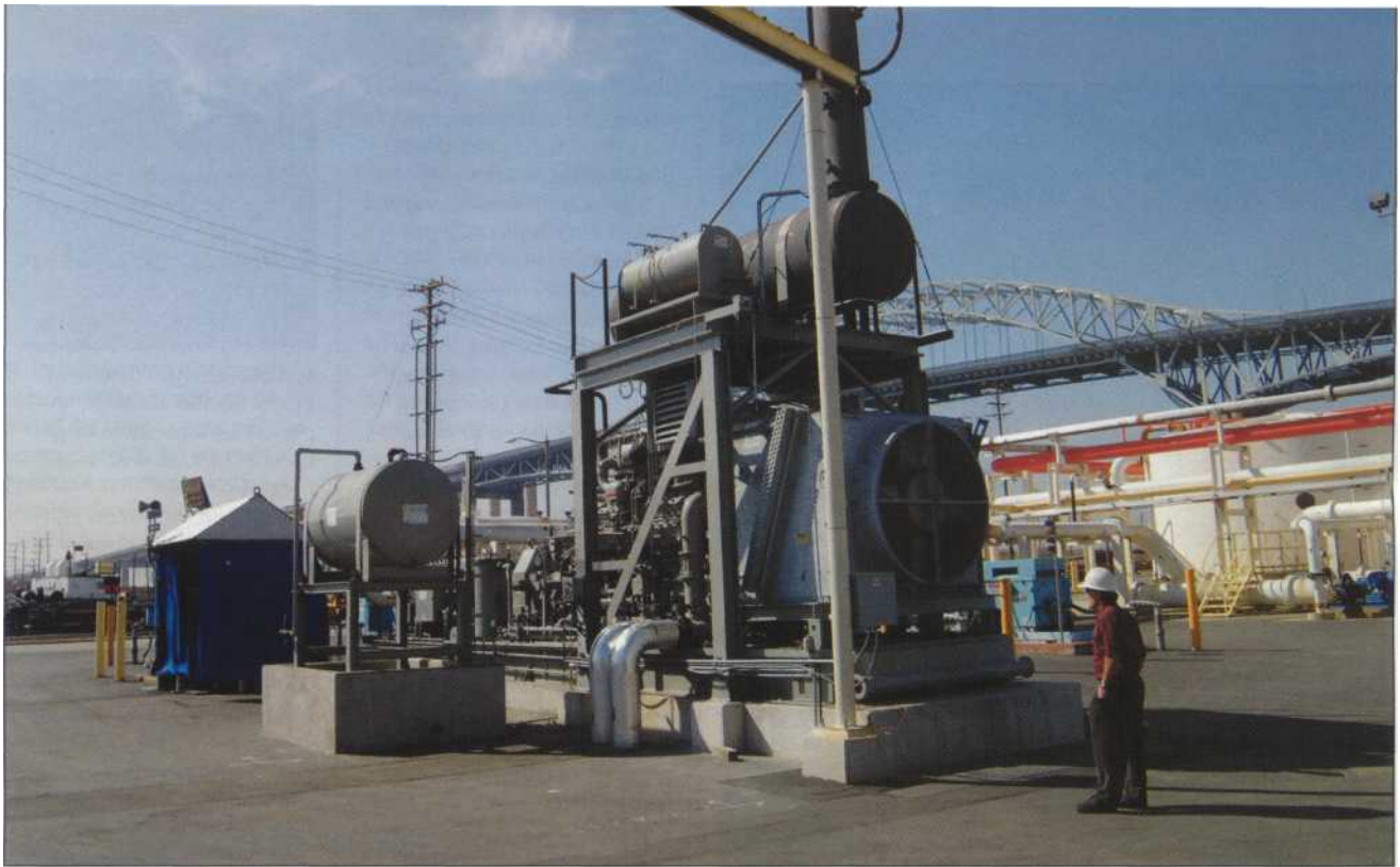
■ Tidelands Oil Production Company installed a Waukesha VHP P9390 GSI engine and pump package. The 2000 hp (1491 kW) natural gas-fueled engine drives a high-pressure centrifugal pump that's being used to inject water into several old oil reservoirs. The package replaced one of three electric motor-driven units previously used.
