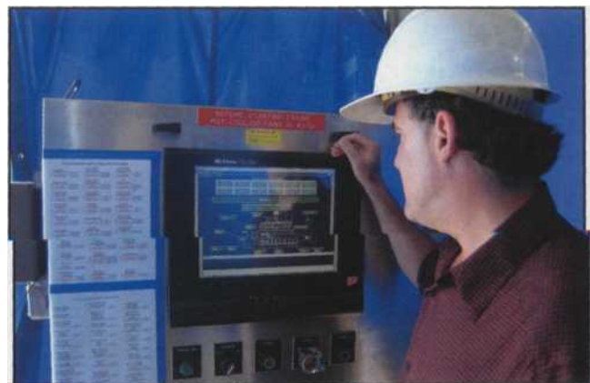
■ The entire engine and pump package uses a GE/Fanuc control system for overall control and monitoring functions.
