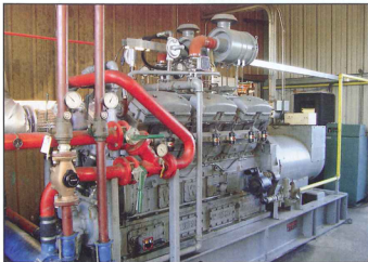
The California Emission Commission field test of the Continental Controls Corp. (CCC) ultra-low emissions system utilized a Waukesha L3711 engine.
